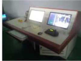
PLC控制及远程监控室 PLC Control and Remote Monitoring Room
